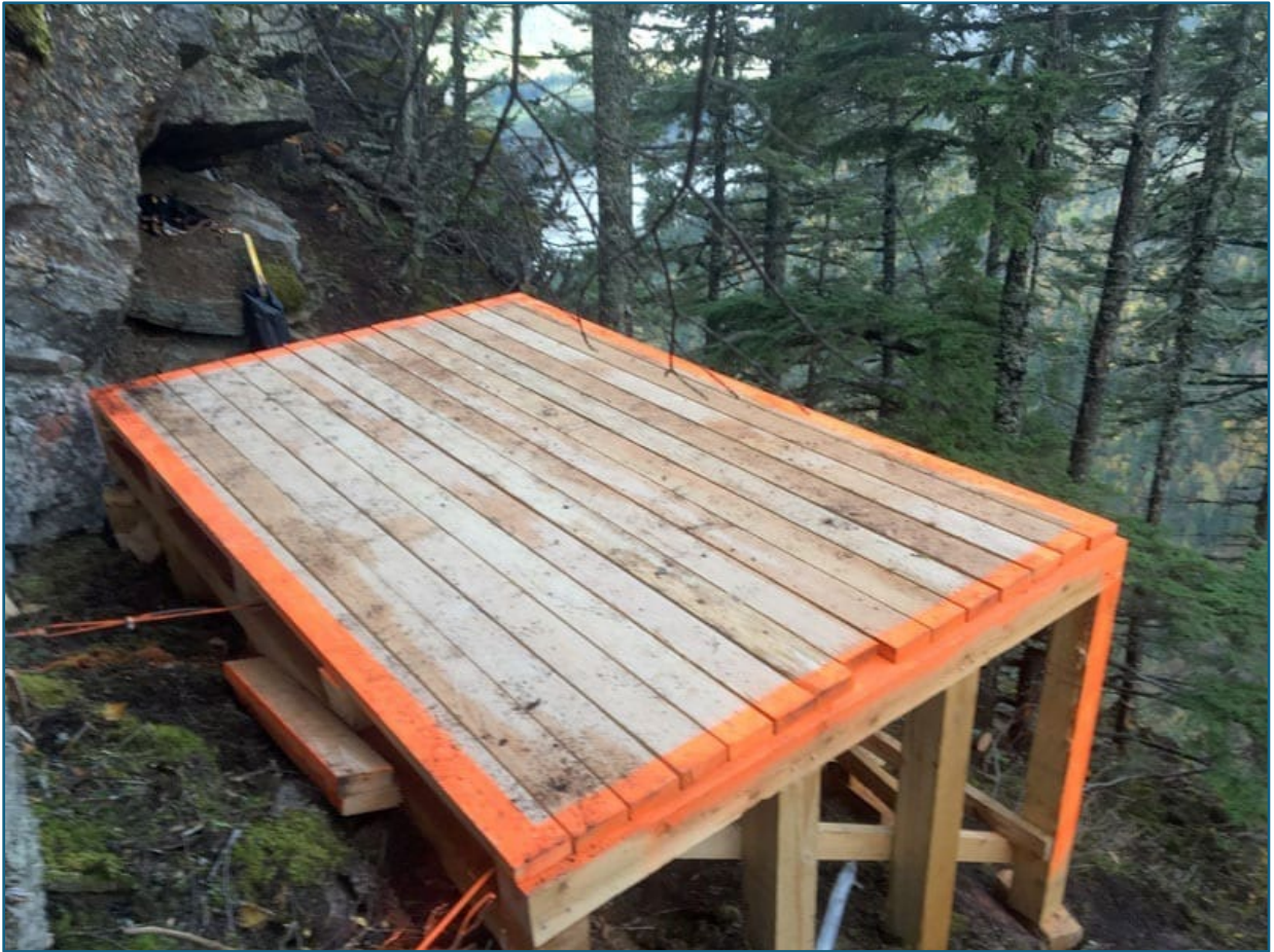
Figure 4. Engineered timber pad for staging drilling equipment (e.g. water pump relay station).
