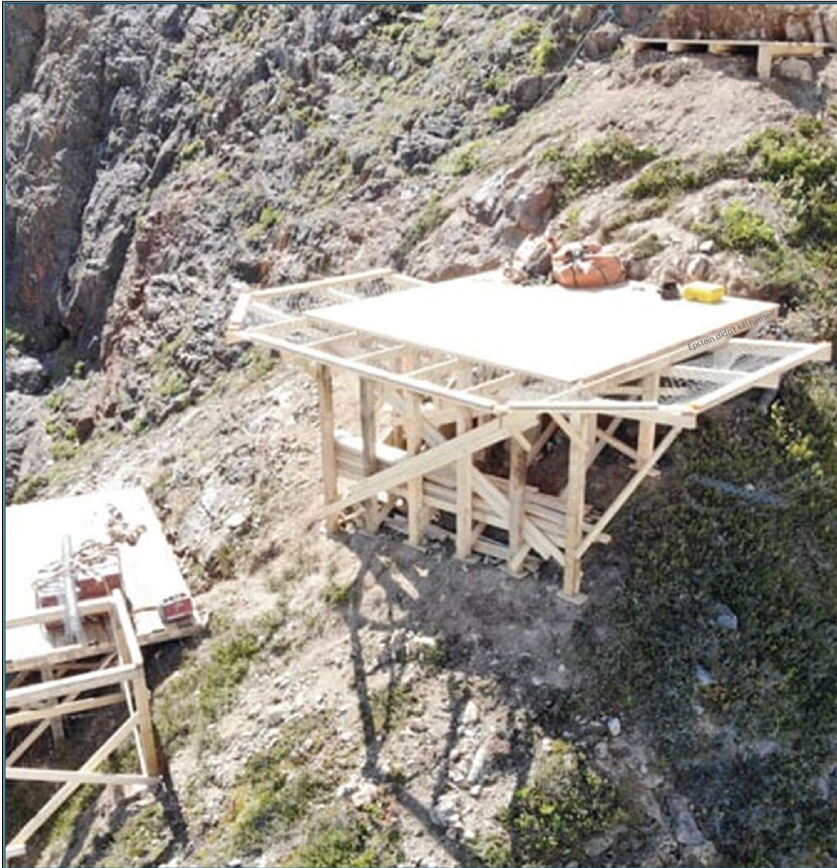
Figure 1. Engineered timber pads. Note the lack of excavation, minimal surface disturbance, wooden footers and “aircraft carrier” fall protection.
