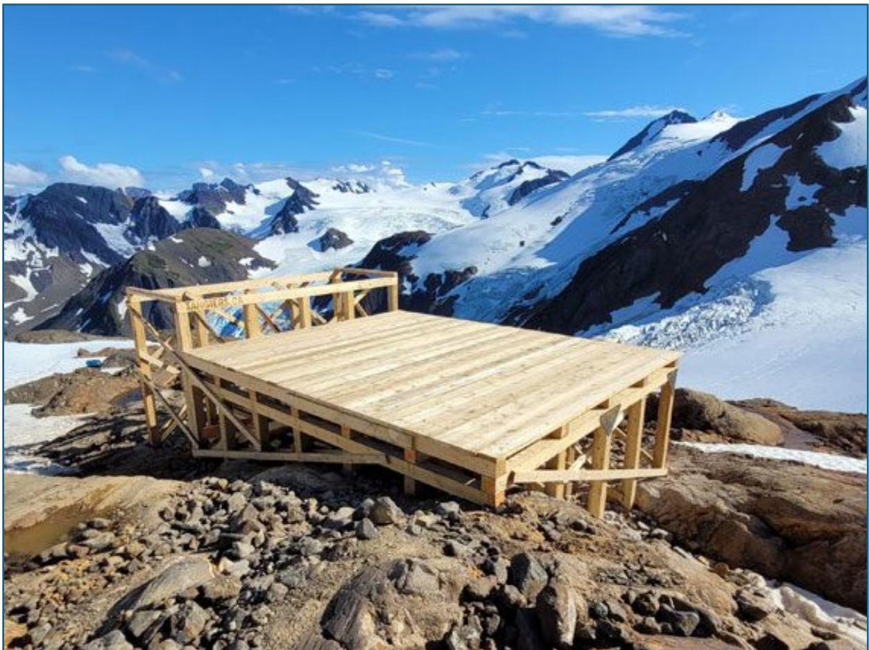
Figure 2. Engineered timber pad with rod rack for drilling equipment staging. Note the lack of surface disturbance in rocky terrain. Road-accessed sites may have a similar timber pad for water and equipment staging.
